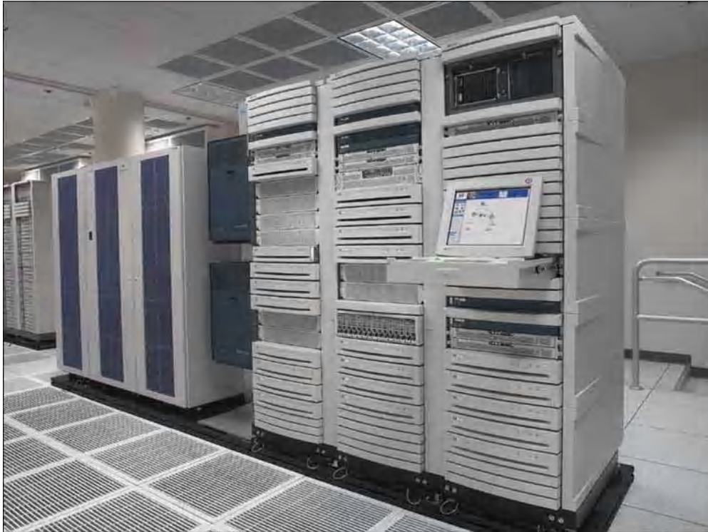
Figure 4: Control racks of the Utility Data Center (HP Labs, Palo Alto, Nov 2004).
